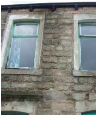
General disrepair before
